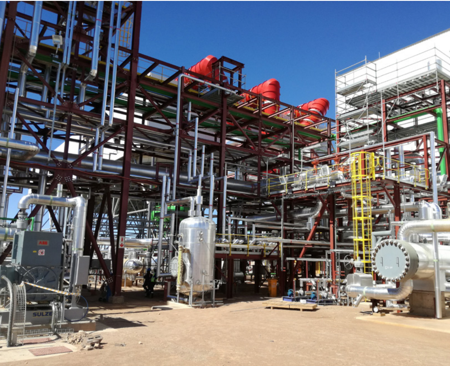
South Africa . 2015 . Xina Solar Plant ©2017. African Development Bank Group
