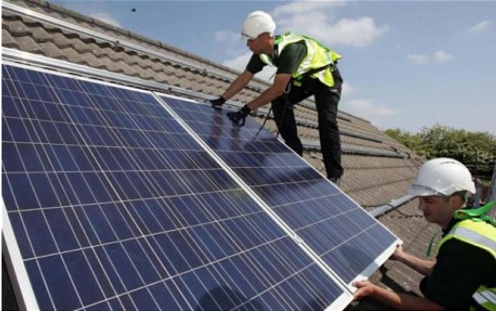
Workmen installing solar panels on to the roofs of homes Photo: PA
