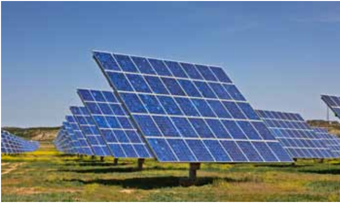
Illustration 7. A solar array
